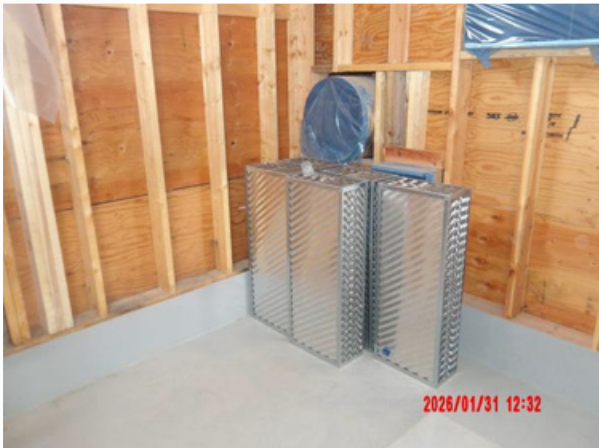
HVAC installed in therapy penthouse
