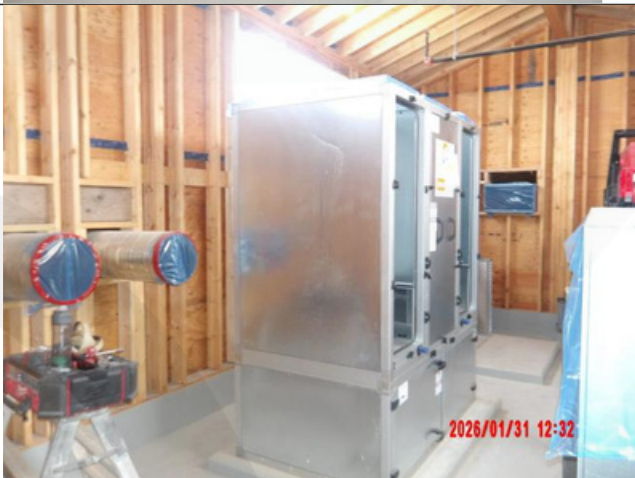
HVAC installed in therapy penthouse
