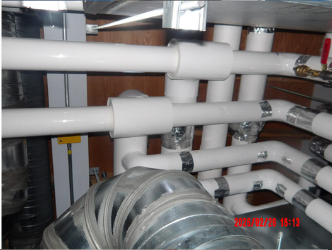
Pipe insulation West residence penthouse
