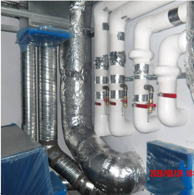
Duct wrap & pipe insulation, West residence penthouse
